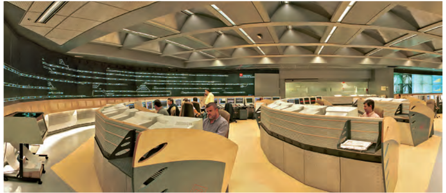
Metro control post at the Alto del Arenal station
